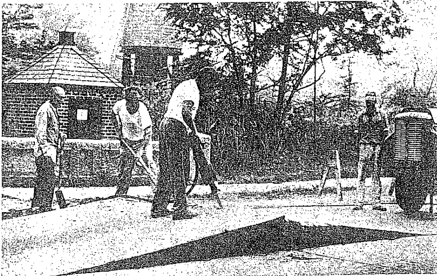
FIG. 9.12. A road that buckled because of expansion during the summer heat. (Courtesy of the New York Department of Transportation.)
